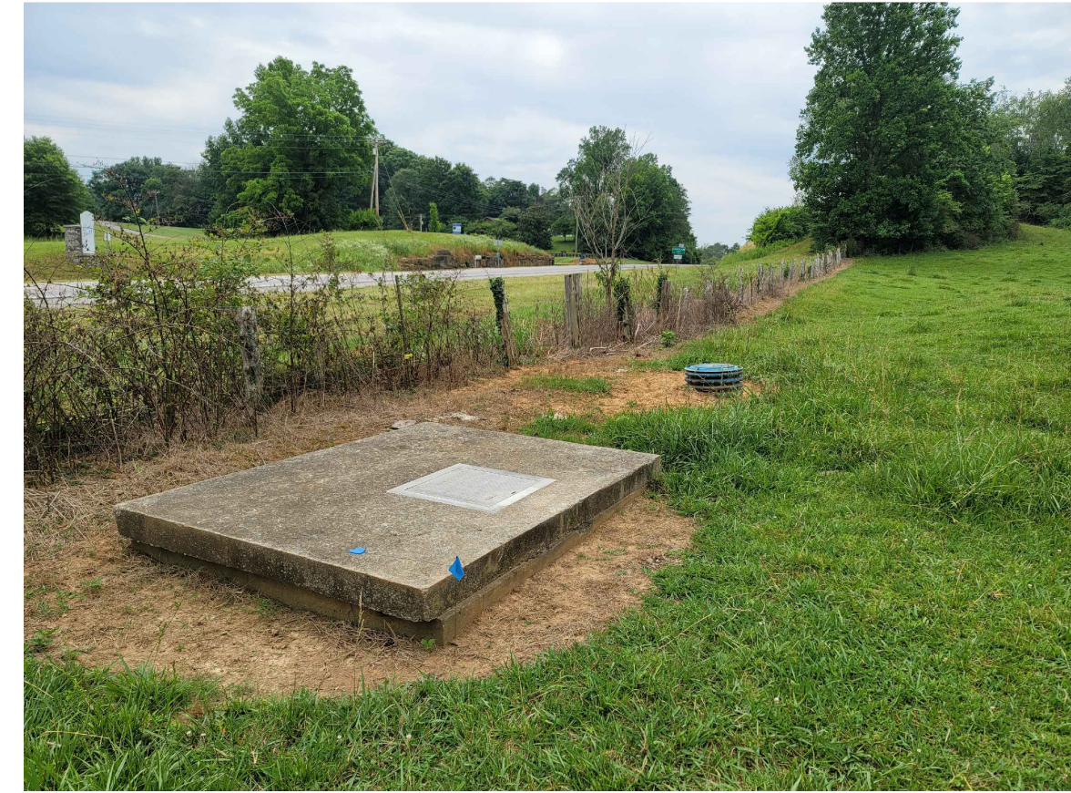
METER 11: EX. METER (TO BE REPLACED) FACING SW PHOTO 11 NOT TO SCALE
