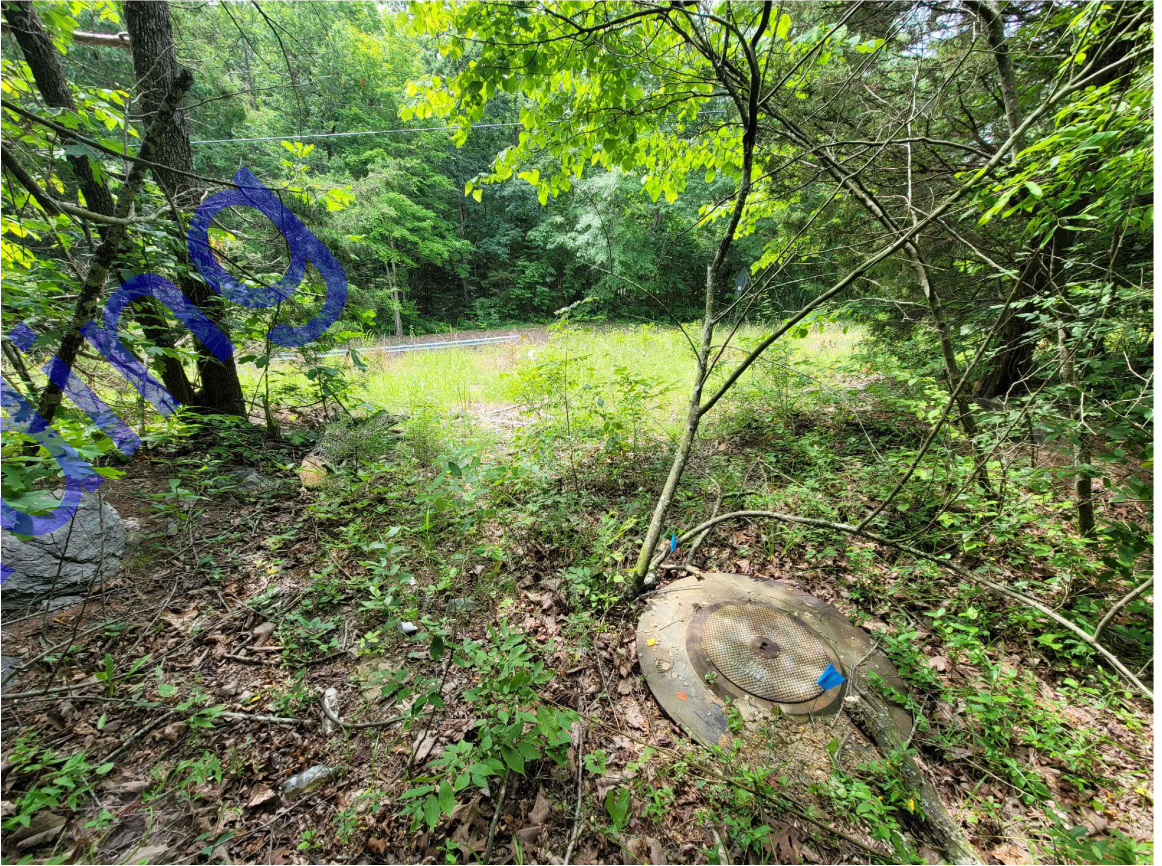
METER 1: EX. METER (TO BE REPLACED) FACING SE
