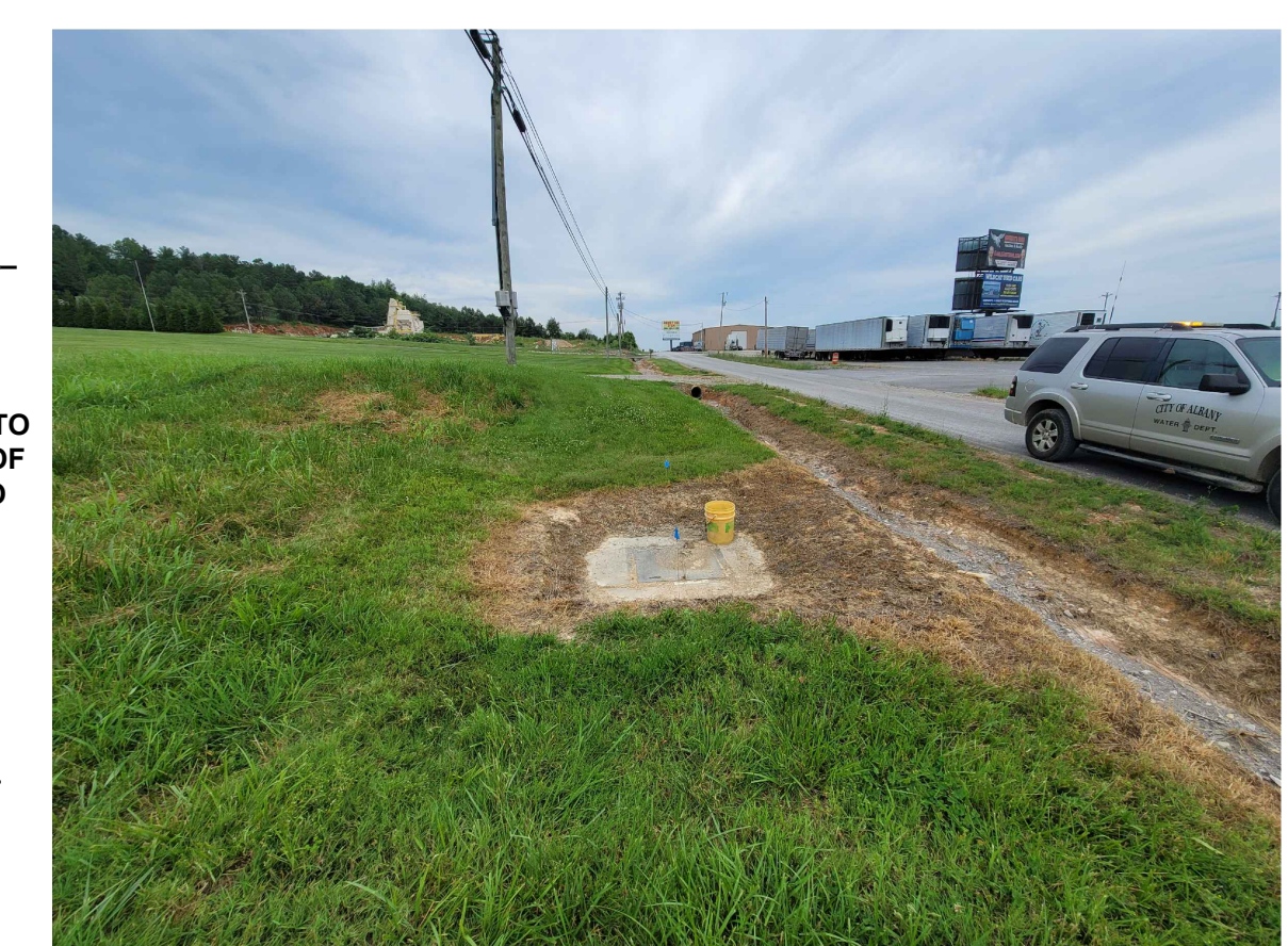
METER 36: EXISTING METER (TO BE REPLACED) FACING NORTH PHOTO NOT TO SCALE 36
