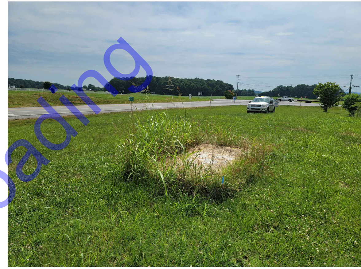
METER 10: EX. METER (TO BE REPLACED) FACING EAST PHOTO 10 NOT TO SCALE
